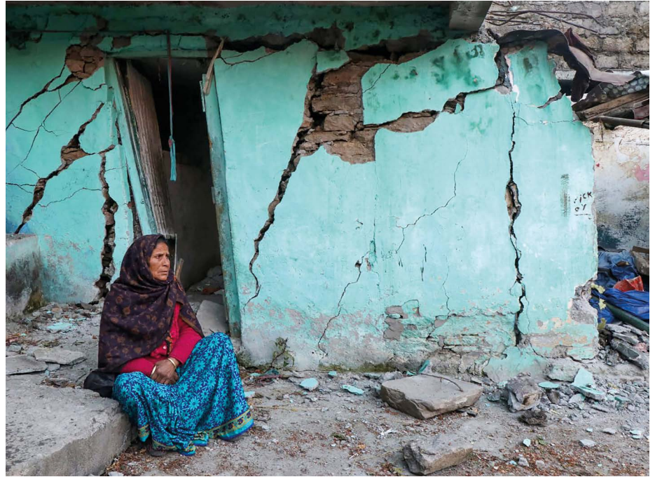
In Joshimath, India, cracks developed in homes in January 2023 as the town began to sink.
